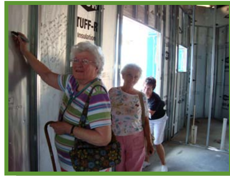
Good Shepherd Hospice volunteers leave messages of support and hope on the unfinished walls of the Bud and Donna Somers Hospice House in Sebring. From left: Marge Stella, Elaine Short and Joan Schumaker.
